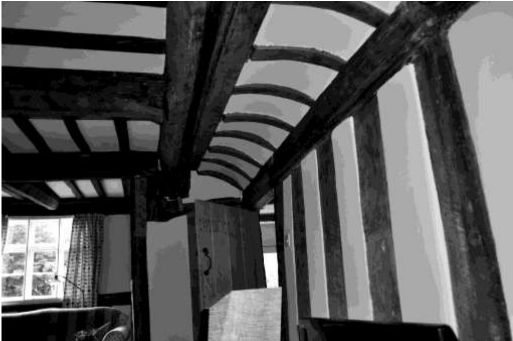
Figure 6. The Old Maidenhead, Lyonshall. This shows the internal jetty with coving on the right and the inserted counterchange ceiling on the left
