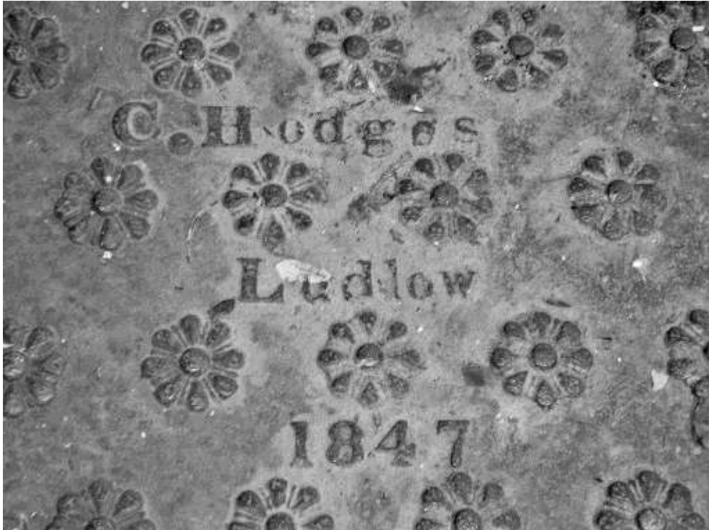
Figure 3. A dated cellar flap outside 18 Etnam Street, Leominster, cast by Chaplin Hodges of Ludlow in 1847, at about the period when his Hereford foundry was established
