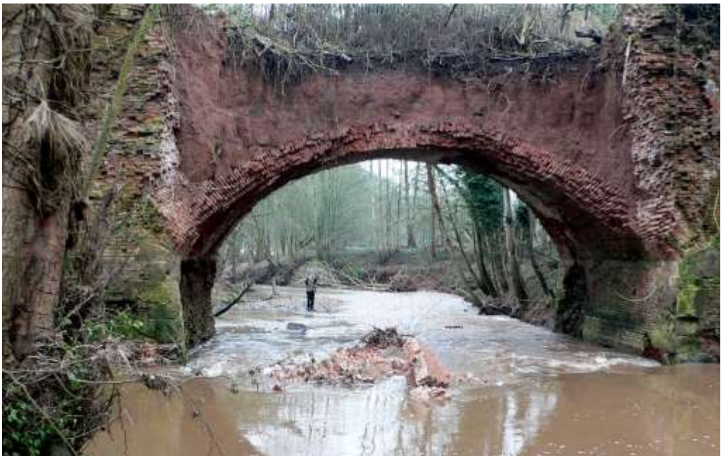
Plate 4.2. The upstream face of the Rea aqueduct after face collapse, 10 March 2013. (©G. Calderbank)
