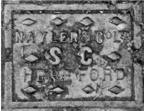
Figure 4. A stop-cock cover, at the entrance from Castle St. into the Cathedral Close, cast by Nayler and Co. Ltd.
