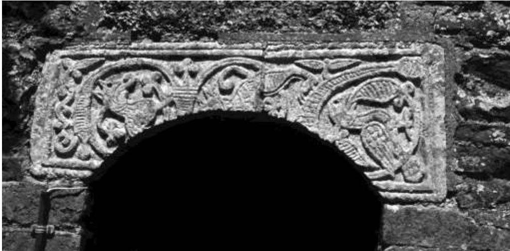
Figure 1. Acton Beauchamp: an early-ninth-century cross-shaft ‘reused as a lintel’ above the south doorway into the tower. Note the crack in the middle of the lintel (J. Hillaby, 2013)
