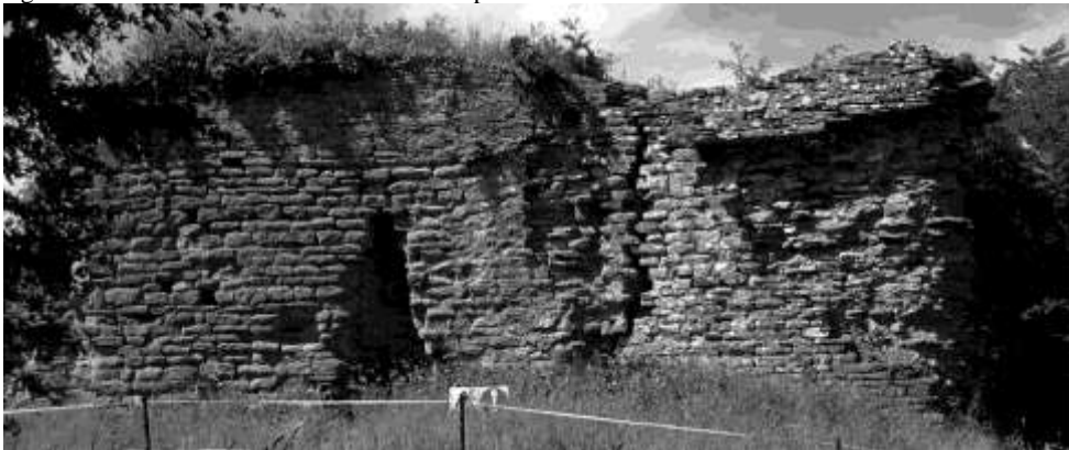
Figure 6. The same wall in 2008 showing the gradual deterioration
